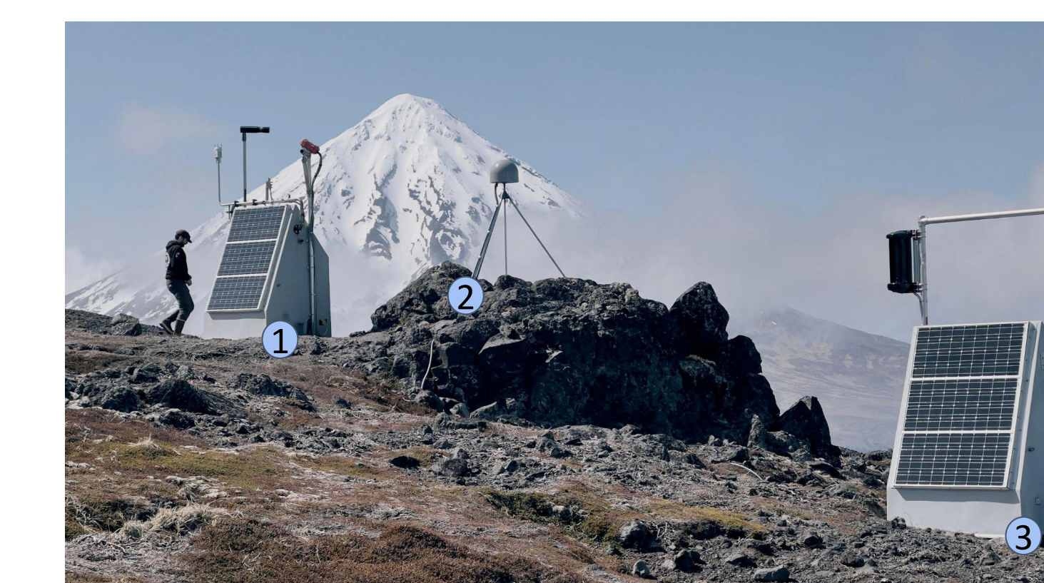
A Multi-disciplinary station on Cleveland Volcano, AK (Carlisle Volcano in the background). The overall system includes multiple Centaur Networked Dataloggers (1), the system also includes Seismometer (Trillium Compact), GNSS Reference Receiver (2), and Triaxial Magnetometer measurements. The secondary hut (3), includes camera systems to monitor the plume. Photo: Bacon, Conor Image courtesy of the LDEO / Columbia
