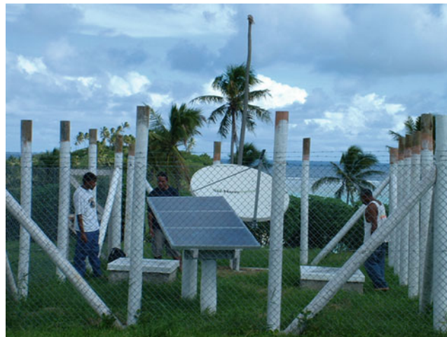
Fig. 7 Rural vault installation with satellite communications in Fiji
